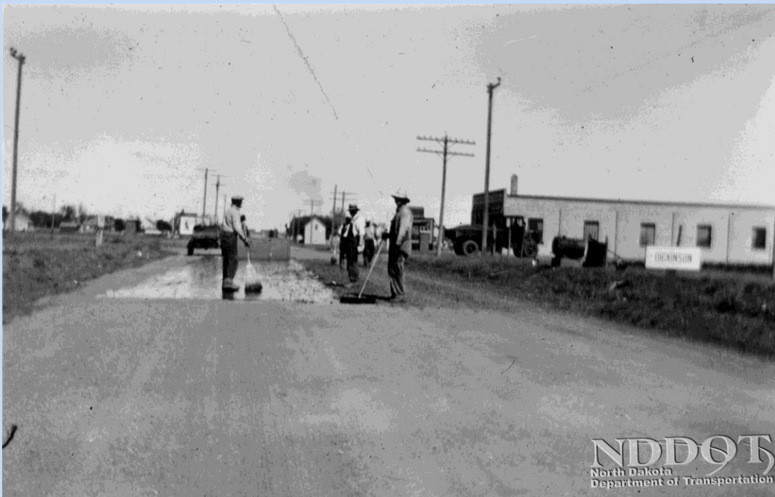
North Dakota State Highway Department crew patching U.S. 10 on the west edge of Dickinson in the 1920s.
